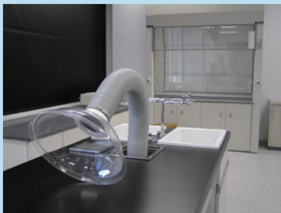
A local exhaust ventilation system is placed in the new experiment laboratory. A fume hood is on the back. Electronic balances and spectrometers will be placed on the left table.
